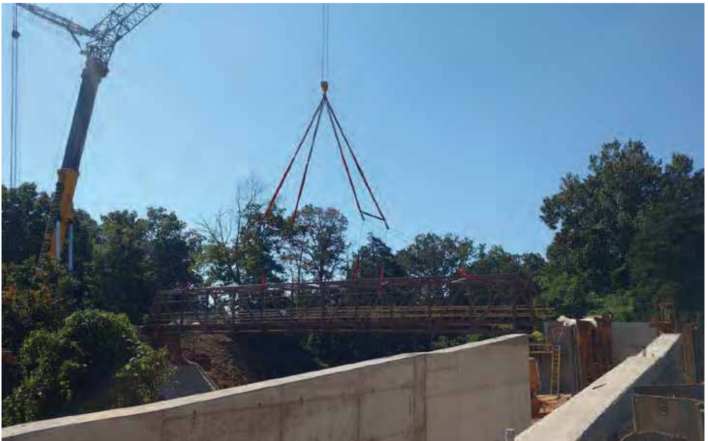
Construction of McIntire Park shared use path bridge, Photo: City of Charlottesville
